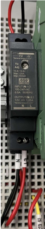
Power Supply Whole View
