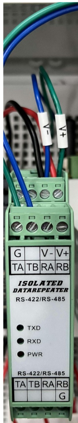
Wiring Connection-Upper Side
