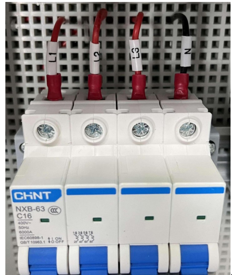
Wiring Connection-Upper Side
